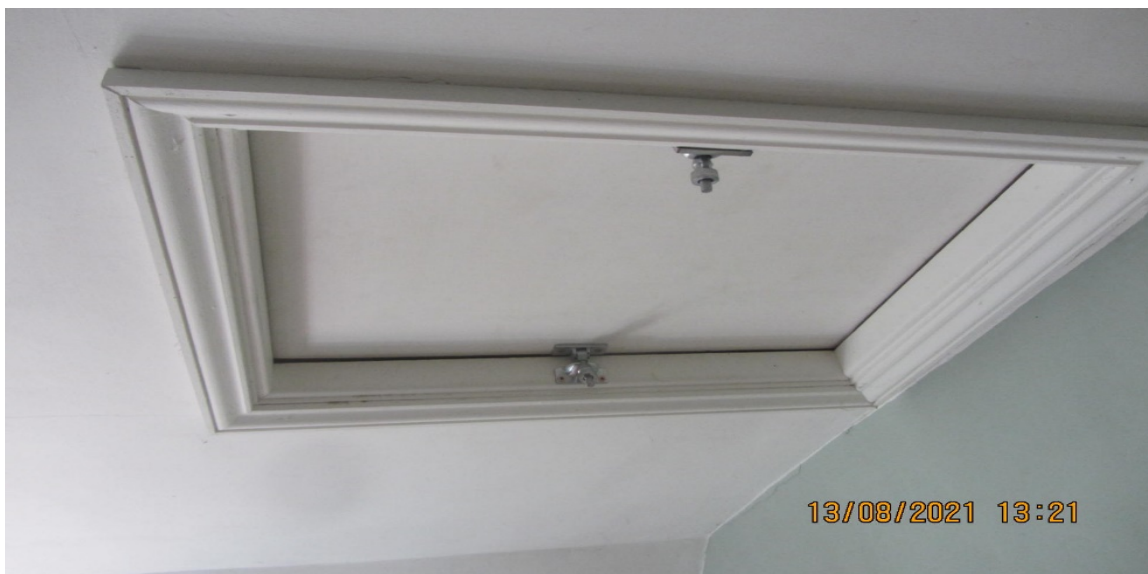
Figure 7: Loft hatch fitted with Brighton latches and rubber strip to make an airtight seal.
