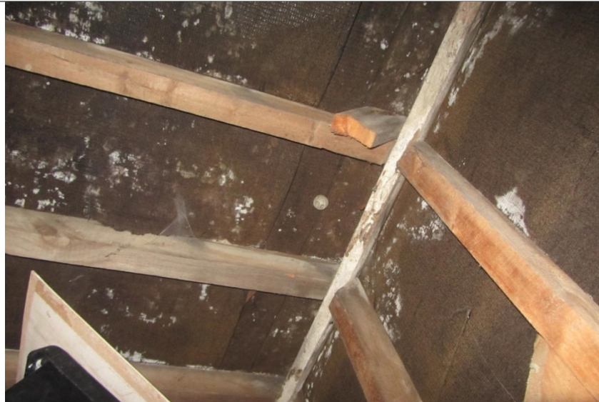
Figure 3: Mould on roof felt
