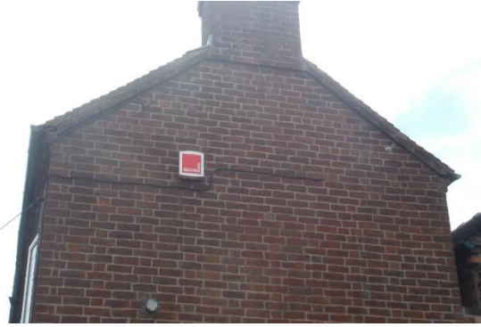
Figure 19 Gable end with insufficient overhang for EWI
