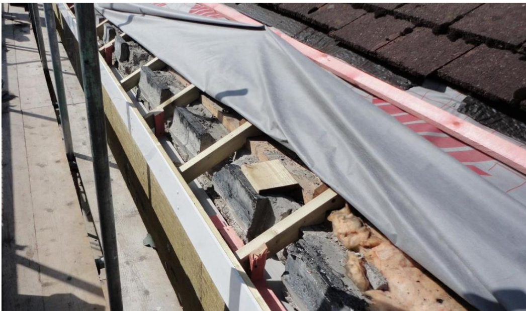
Figure 7 Roof eaves being extended example (Ref BRE External Wall Insulation (EWI) Report P107357-1000)
